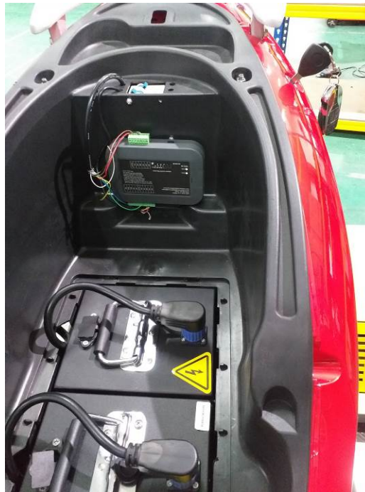
Figure 10 : Logger (gray box at top) installed in battery bay. The two batteries can be seen in the foreground.
